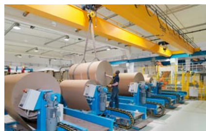
Overhead travelling crane above the packing machine
